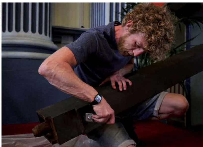
▲ Pipework has not been altered in any way; trainee Joe Calder works on site
